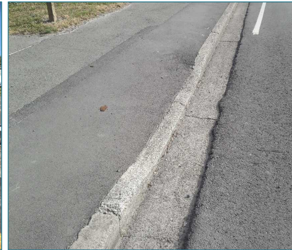
Poor example of kerb ramp
