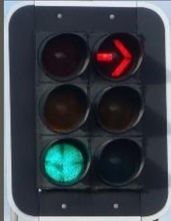
General traffic signals
